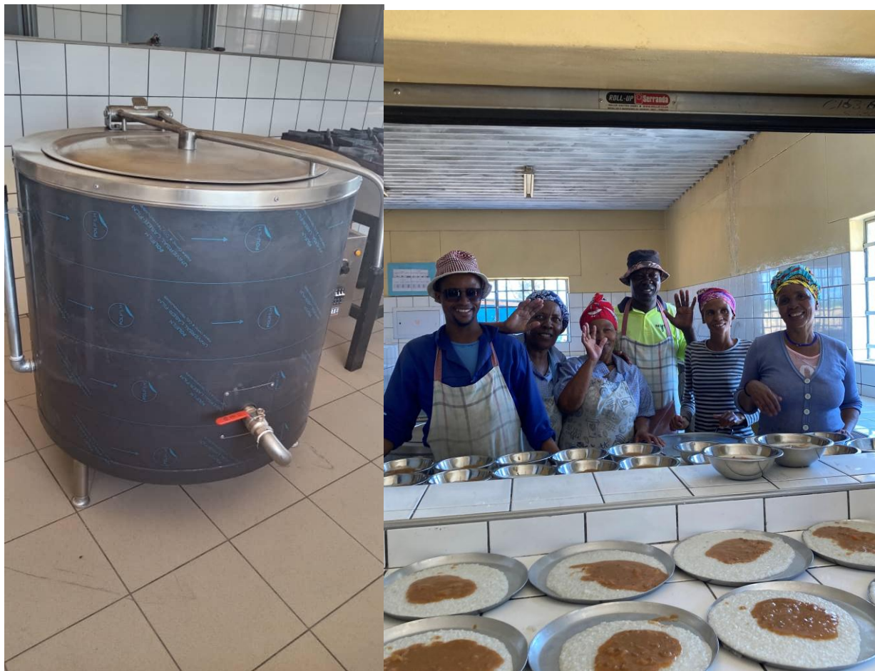
The new electrical cooking pot and the happy canteen staff.
